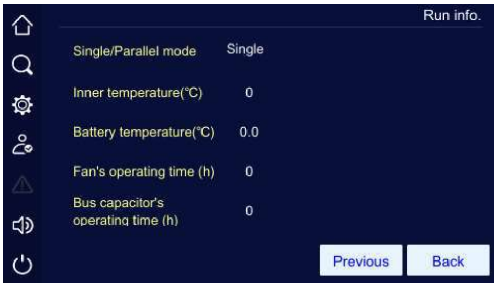
Working status page 2 (single UPS)
